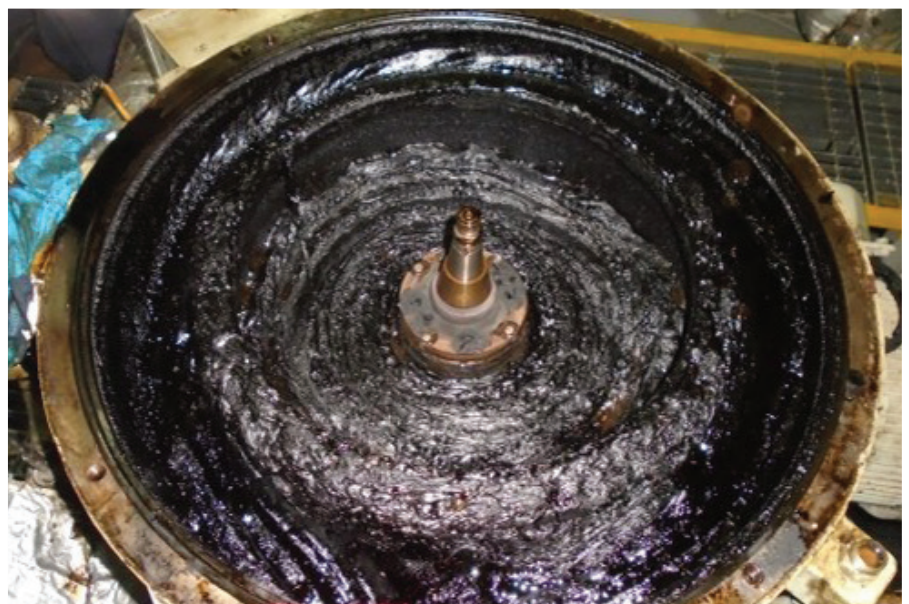
Fig. 34: Heavy sludging and block separators as a result of either unstable fuel or incompatibility between two fuels.
